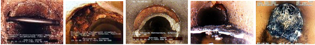
Pipes damaged by different reasons
