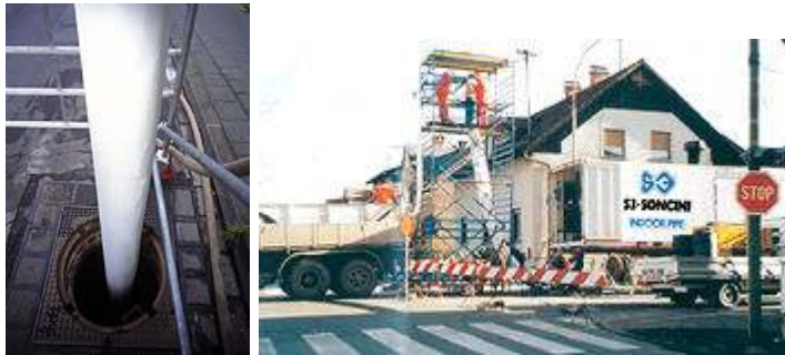
Installation of equipment without obstructing the circulation
